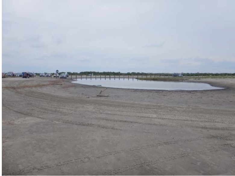
Passage from Elmer's Island parking lot to the Gulf after scouring by Hurricane Zeta. Taken 5-29-21.
