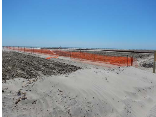
Bird nesting abatement windrows. Their purpose was to Discourage birds from nesting during construction. 4-10-16.
