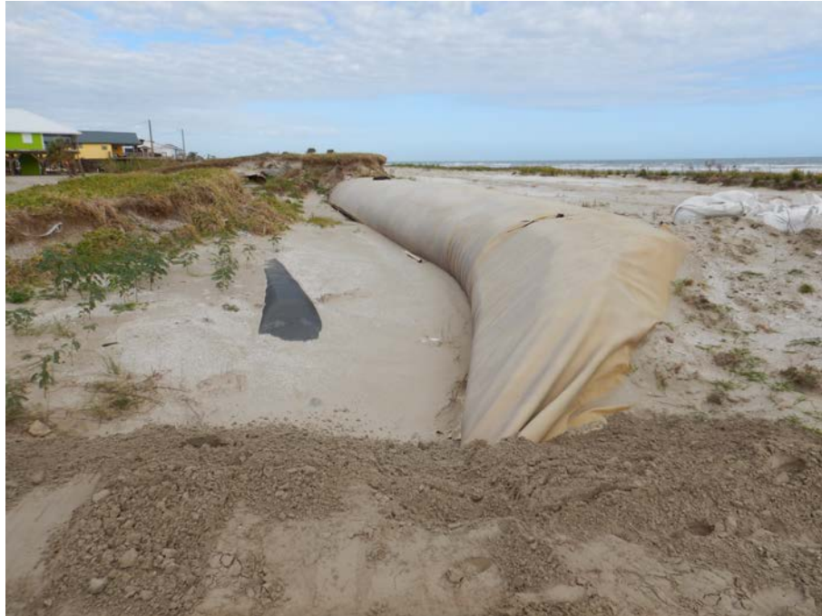
“Burrito” levees were unearthed in the overall levee systems on Grand Isle in Hurricane Ida. Taken November 19, 2021.
